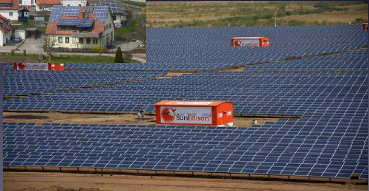
600 MW Solar Powerplant, Gujarat
