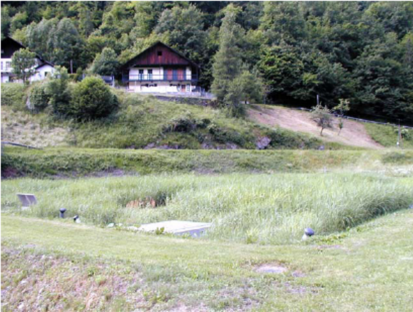
Queige (73) – 500 p.e. – Phragmifilter® wastewater treatment plant
