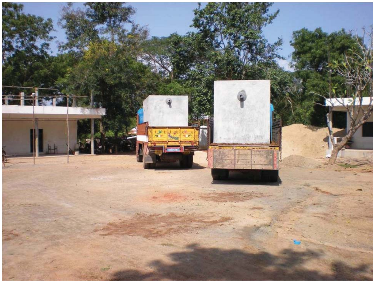
Kadambadi settlement, 2008 183 households 43 prefab dewats modules
