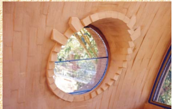
Building a bull eye, 80 cm dia Catenary vault, 6 m span, 3 m rise with the Free Spanning technique
