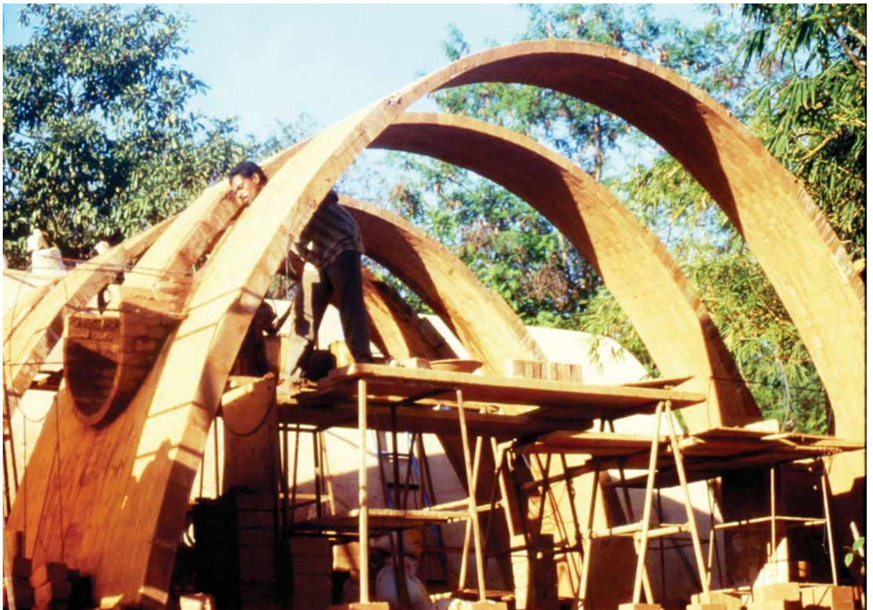
Building a catenary vault, 6 m span, 3 m rise with the Free Spanning technique
